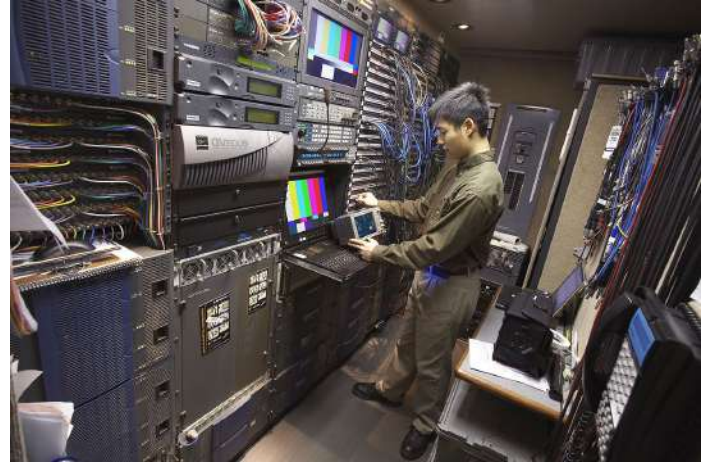
WFM5200 Compliance Checking in distribution or broadcast applications.
